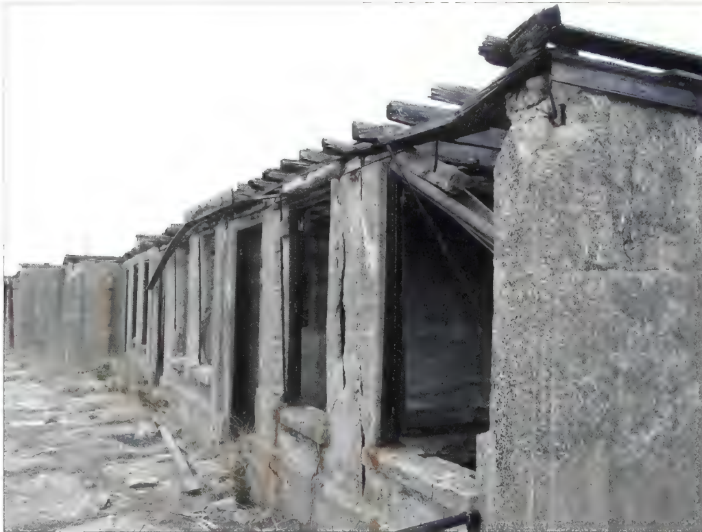
Figure 3.27. Fire control stations, Battery Potter. On the terreplein, two groups of deteriorating concrete structures are located west of the former gun emplacements. The structures served as fire control stations and feature large openings in their east elevations to provide views to the Atlantic Ocean (Olmsted Center, January 2009).
